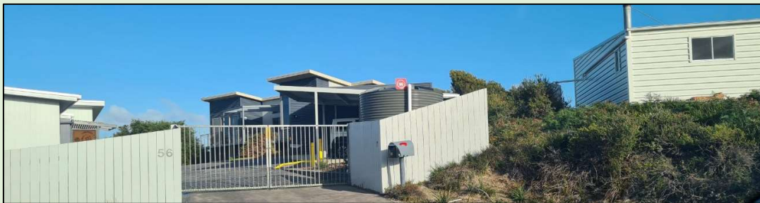
Figure 12: Firefighting tank at 56 Seascape Drive.
