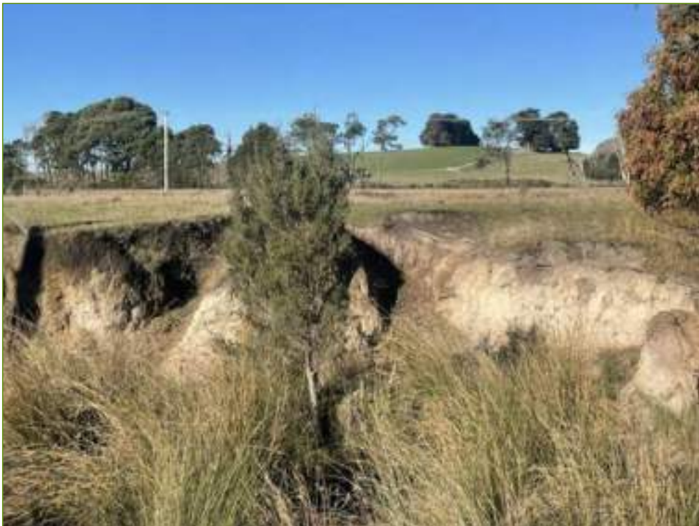
Figure 21 The watercourse is characterised by high stream banks and a wide floor, unsafe for livestock to negotiate. Taken at site assessment 29/5/2025.
